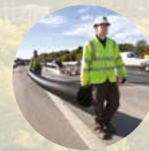
Surface Water Drainage
