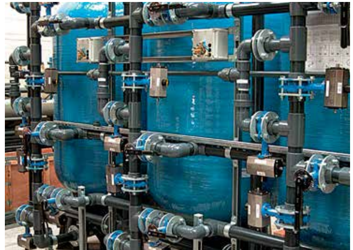
Picture supplied courtesy of Sterling Hydrotec.
